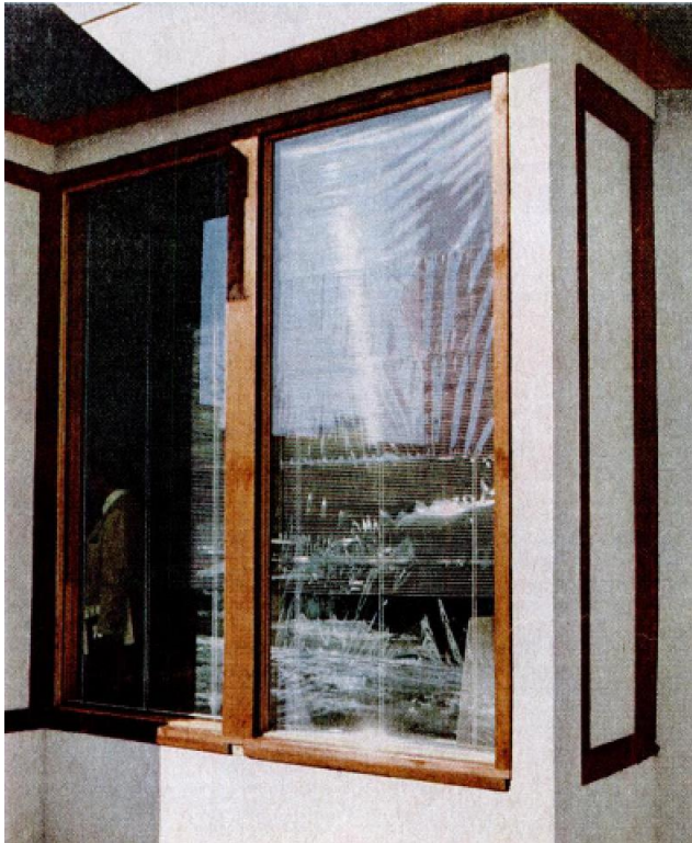
Mirror Blinds Reflect Sunlight to the Ceiling
